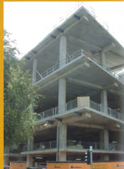
The striking North West corner of the new GPO Structure at the corner of Elizabeth Street and Little Bourke Street. Note the requirement of a cantilevered floor in two directions.
