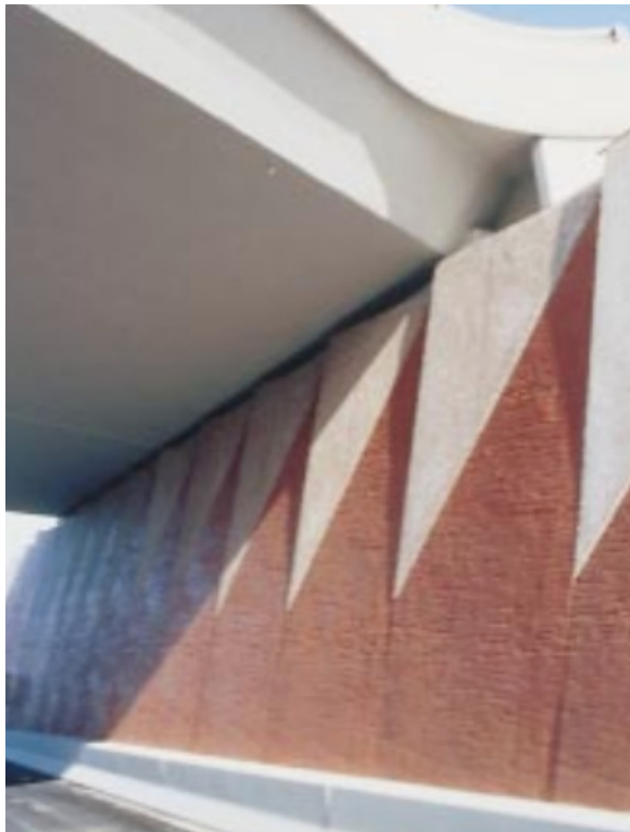
Patterned precast retaining wall units on Melbourne Freeway project using 7.6% deep marigold oxide
