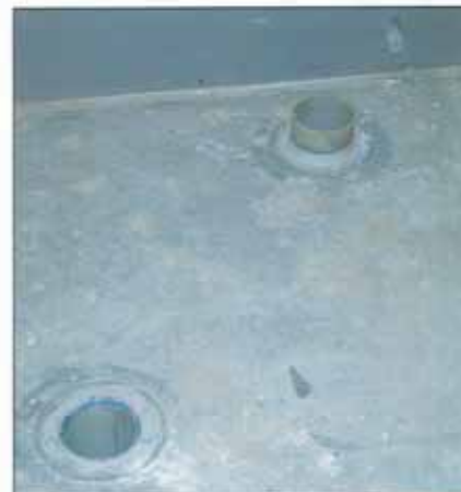
FLOOR PENETRATIONS FOR WASTE PIPES WERE CORED ON SITE AND SEALED AGAINST FIRE PENETRATION. CORING ON-SITE IN THIS INSTANCE GAVE GREATER FLEXIBILITY OF FLOOR PANEL USE. IN OTHER INSTANCES IT MAY BE MORE EXPEDIENT TO CAST ALL SERVICES INTO THE UNIT AT THE PRECAST YARD. ■
