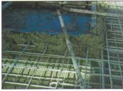
PLACING A GREEN-TINTED CONCRETE VENEER FOR A LARGE WALL PANEL; NOTE VENEER TURNED-UP AROUND WINDOW REVEALS PRIOR TO THE PLACEMENT AND COMPACTION OF THE STRUCTURAL, GREY CONCRETE BACKING.
