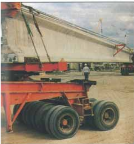
EXAMPLE OF LATERAL STABILITY BRACING FOR 35-m GIRDER USING TENSIONED CABLE TIES.
