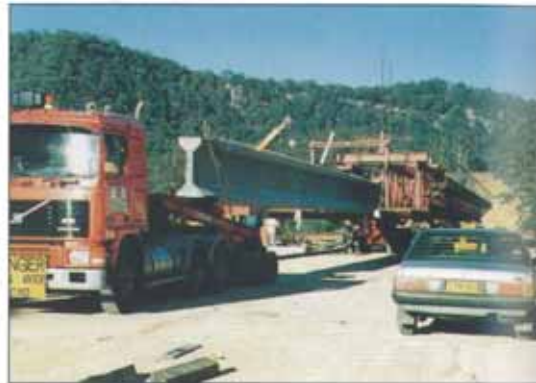
35-m-LONG, TYPE 4 PRECAST BRIDGE GIRDER WEIGHING 40 TONNES BEING POSITIONED FOR LAUNCHING, MITTAGONG BYPASS, NSW.
