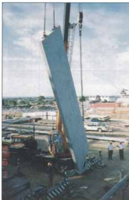
PANEL, TRANSPORTED HORIZONTALLY, USING AN 'A' FRAME SUPPORT BEING ROTATED TO THE VERTICAL USING ROLLING SHEAVE RIGGING SYSTEM.
