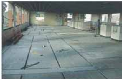
CONVERSION OF WAREHOUSE TO APARTMENTS. PANELS WERE PLACED THROUGH EXISTING OPENINGS IN THE BUILDING FACADE WITHOUT REMOVING THE ROOF. SHEAR KEYS TO BE GROUTED; NO INSITU TOPPING REQUIRED.
