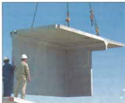
WALL AND ROOF UNIT BEING LIFTED. AS VIEWED, THE UNIT WILL BE REVERSED THROUGH APPROXIMATELY 180° WITH THE LEADING EDGE OF THE ROOF LOCATED ON THE CORBEL, VISIBLE ON THE IN-PLACE UNIT.
