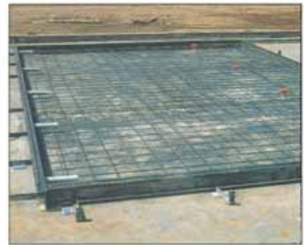
ON-SITE CASTING – FABRICATED STEEL EDGE MOULD, REINFORCEMENT, ETC IN PLACE. BED TO BE CLEANED BY AIR-BLASTING PRIOR TO CASTING CONCRETE.
