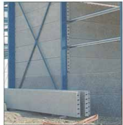
TECHNICAL AND WAREHOUSE FACILITY. HORIZONTAL, EXPOSED-AGGREGATE-FINISH PANELS. NOTE USE OF DARK RIVER GRAVEL IN BOTTOM PANEL TO SUGGEST PLINTH.
