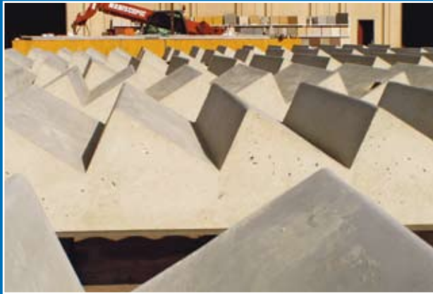
Manufacture of precast components can commence as soon as drawings are approved.
