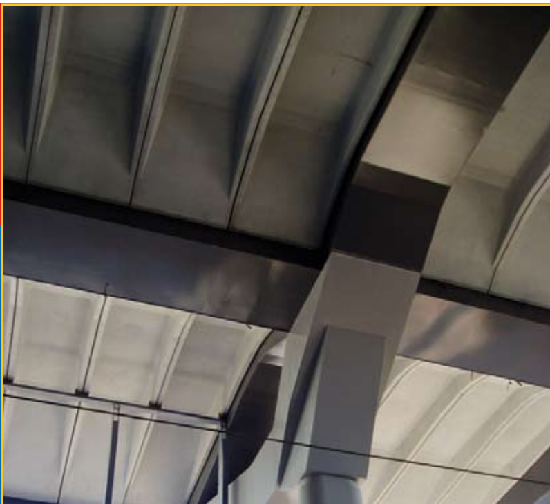
The blemish free off-white precast flooring segments also serve as a coffered ceiling.
