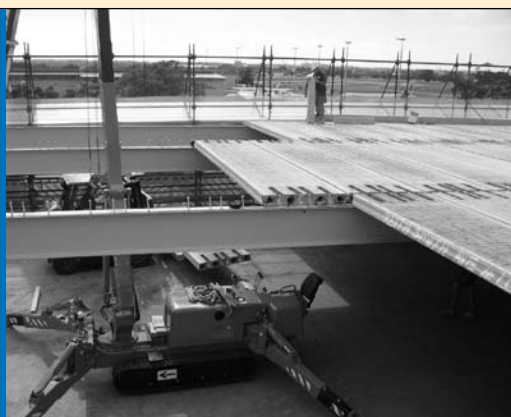
Figure 2 (a): Erection of hollowcore (manufactured by Rescrete Industries) at Sydney Airport, Domestic Terminal Carpark
