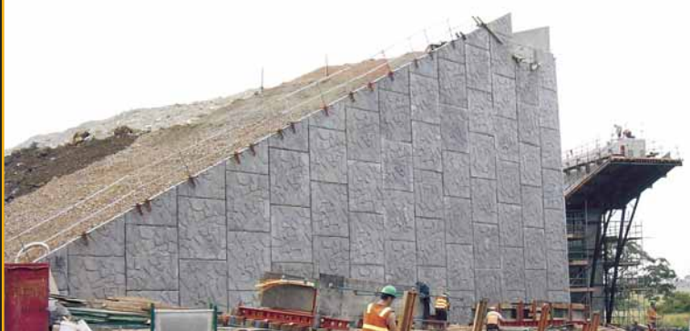
Reinforced Earth wall with random bluestone rock finish at Merri Creek Bridge
