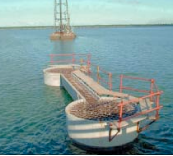
View of hollow precast pilecap and tie beam shells before the introduction of insitu concrete. Reinforcement was detailed to allow placement of prefabricated cages.
