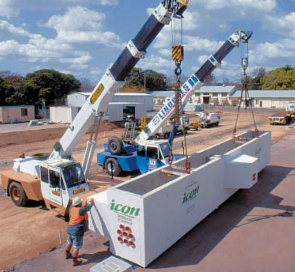
Double lift of one of the 23 tonne cable jointing pits at the Kelvin Grove site.
