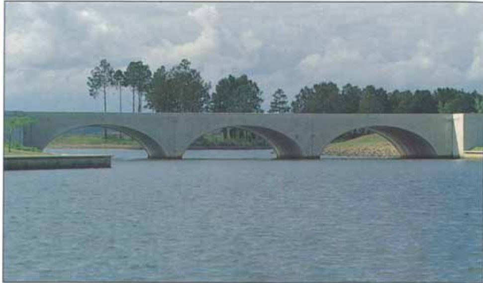
MULTIPLE-SPAN APPLICATION. NOTE THE ARCH CURVE IS PROVIDED WITH A CAST-IN CONTINUOUS NIB TO SUPPORT MASONRY VENEER IF REQUIRED.
