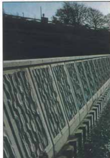
DOLOS UNITS BEING CAST, PORT BOTANY. SEAWALL, BEYOND LINE OF BROADWALK. USE OF FORMLINERS TO CREATE VISUAL INTEREST AT FACE OF PANEL - FLOOD-PROTECTION WALLING.
