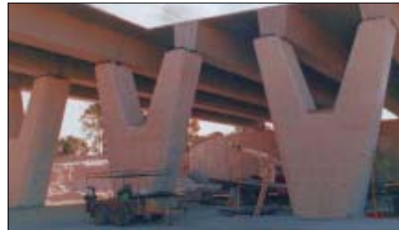
Spencer Road Bridge under construction; featuring three unique Y-shape columns supporting the 6-girder superstructure
