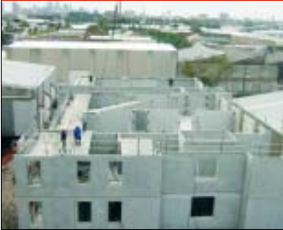
Erection of hollowcore floor planks and Transfloors balcony units on top floor of the Beaconsfield apartments
