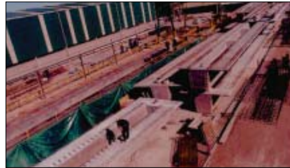
Aerial view of casting yard in Perth where bridge girders for Roe Highway Extension were manufactured
