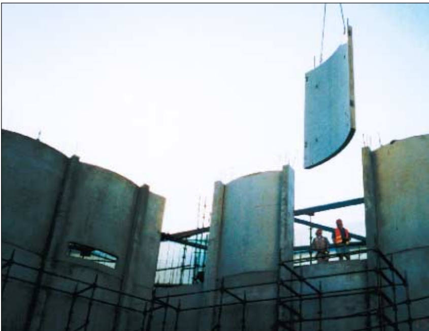
Erection of upper level precast blade columns (top) and erection of 4.1 m high curved panels which form auditorium's main interior walls (above).
