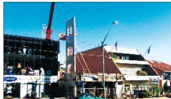
(top) Lifting and turning 3-storey-9.8 m-long wall panel into vertical position and (above) the 9.8 m panel in its final position – seated on ground floor panel; both panels have factory fitted openings for windows and doorway
