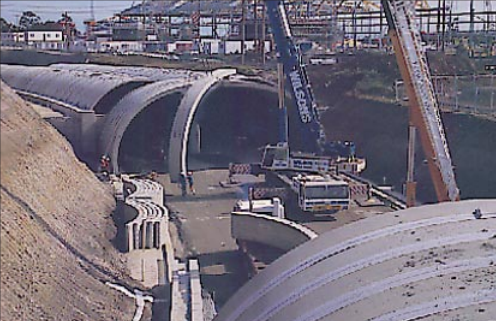
Construction of the Olympic Rail Loop with TechSpan® Arch Tunnels in Sydney
