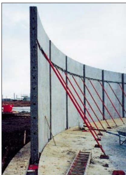
Installation of 3 m high panels to form walling of 45 m dia Clarifier Tank, for Melbourne Water at Werribee Sewerage Treatment Plant
