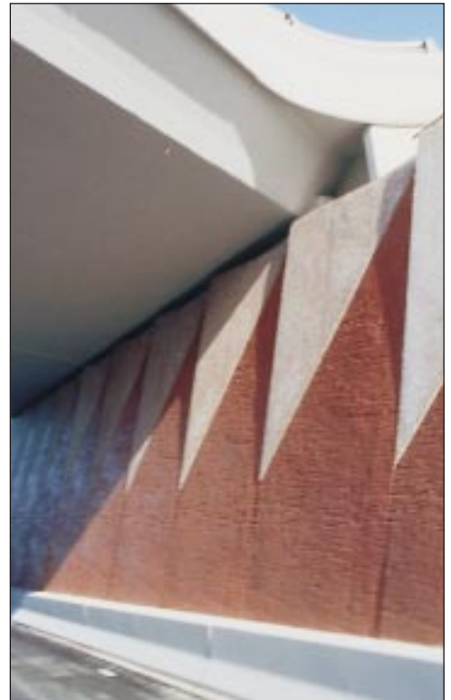
Patterned precast retaining wall units on Melbourne Freeway project using 7.6% deep marigold oxide
