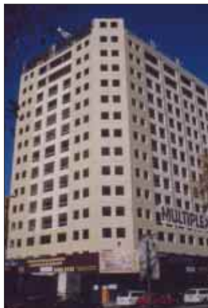
Excelsior Apartments under construction. Builder – Multiplex, GRC supplier – Asurco Contracting Pty Ltd, Adelaide.
