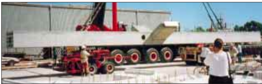
Loading one of the twelve 25 m length, 65 tonne precast columns for the Roxby Downs site
