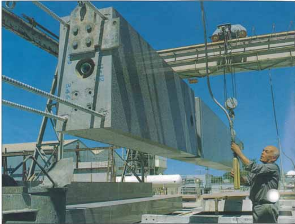
LOADING A 21-TONNE, PRESTRESSED, 12-METRE COLUMN UNIT. THE RECONSTRUCTED GRANITE ELEMENT IS POLISHED ON ALL FOUR FACES.
