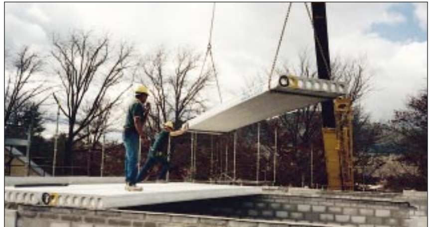
ERECTING 200 mm 8 m SPAN HOLLOWCORE PLANKS ON LOADBEARING BLOCKWORK AT A TOWNHOUSE DEVELOPMENT IN BRADDON, ACT
