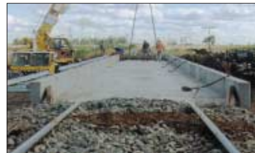
READY FOR BALLAST, TIE AND RAIL PLACEMENT. NOTE CAST-IN RETAINING KERB AND PREFIXED GALVANISED FOOTWAY.
