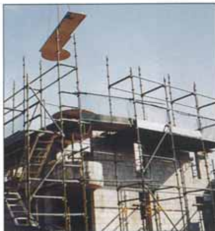
PRECAST HUMESLAB (TRANSFLOOR) BALCONY PANEL BEING LIFTED – NOTE NEAR-CIRCULAR END TO PANEL
