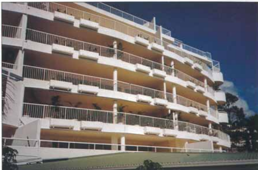
SIMPLE PAINTED FINISH TO THE SOFFIT OF HUMESLAB, POSSIBLE DUE TO THE CLASS 2 OR 3 FINISH PROVIDED
