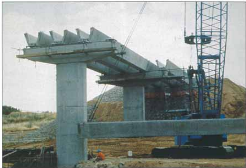
THE RELATIVELY THIN-WALL SECTION OF A PRECAST 'U' BEAM. PLACEMENT OF CONCRETE AND COMPACTION IS AIDED BY THE USE OF A HRWR.
