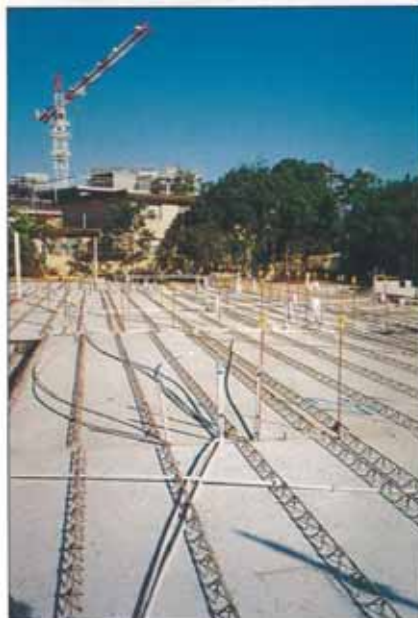
PRECAST PERMANENT, PARTICIPATING FORMWORK IN PLACE. SHOWS CAST-IN TRUSSES, SERVICES IN PLACE, AWAITING TOP, CRACK-CONTROL STEEL AND TOPPING
