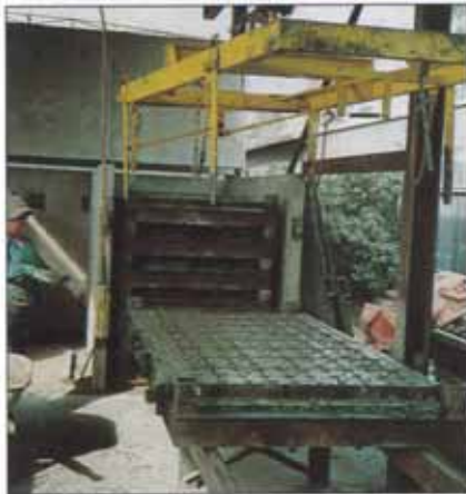
CONCRETE PLACEMENT; SURFACE FINISHED FLUSH WITH SURFACE OF NOZZLE INSERTS. TEXTURED SURFACE FINISH PROVIDED TO GIVE BOND FOR ON-SITE TOPPING. UNIT READY TO ENTER STEAM CURING CHAMBER. THE PRESENCE OF THE PLASTIC MATS AT THE BASE OF THE FILTER SLABS REQUIRED THE PRECASTER TO DEVELOP A CURING REGIME WHICH WOULD ELIMINATE DIFFERENTIAL SHRINKAGE AND THE POTENTIAL FOR EDGE CURLING TO DEVELOP.
