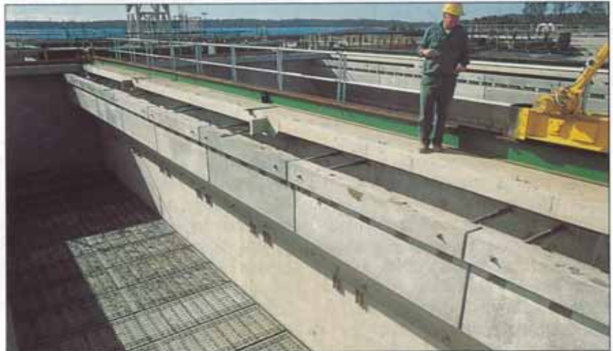
FILTER SLABS, LOCATED ON DWARF WALLS. LAUNDRER UNIT ALSO IN POSITION. PLACING AND FIXING OF THESE LATTER UNITS BY LW CONTRACTING, SPECIALIST ERECTION CONTRACTORS.
