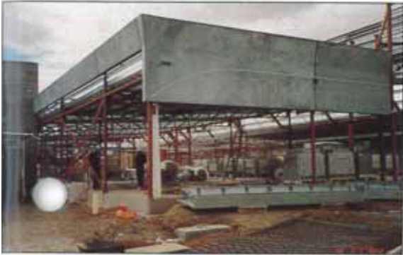
PANELS PARTIALLY ERECTED. NOTE CAST-IN REGLET (THIN LIGHT-COLOURED LINE ON PANEL) TO RECEIVE BULL-NOSED FLASHING OF VERANDAH ROOF.
