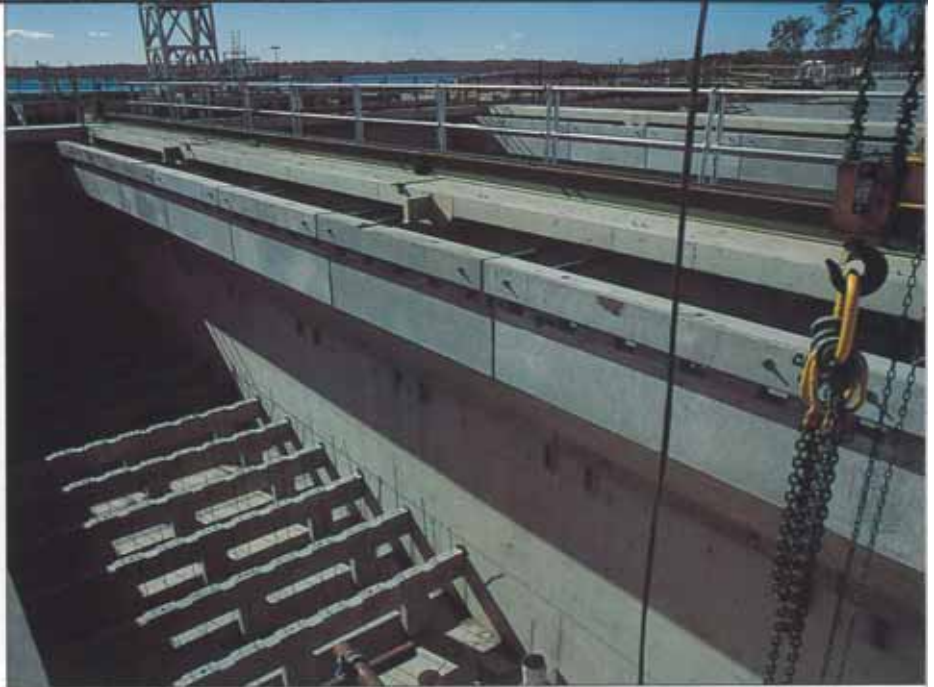
DWARF WALL ELEMENTS BEING POSITIONED. THIS SECTION OF THE WORK WAS UNDERTAKEN BY BARADOM PTY LTD, SPECIALIST ERECTION CONTRACTORS.
