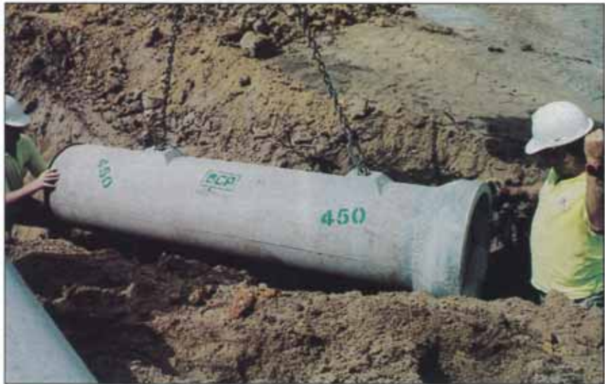
THE USE BY THE COMPANY OF THE REID SWIFT LIFT, ENSURING IMPROVED SAFETY AND EASE OF PLACEMENT.
