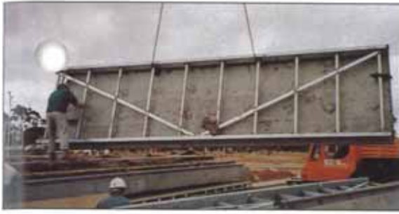
REAR VIEW OF PANELS. STEEL SUB-FRAME FORMED A STRUCTURAL TRUSS, INTEGRALLY CAST INTO THE GRC.
