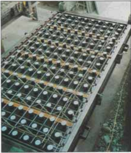
MOULD FOR PRECAST FILTER SLAB; REINFORCEMENT AND MATS OF FILTER NOZZLE INSERTS IN PLACE. JOINTS BETWEEN MATS TAPED. THE PLASTIC MAT AND UPSTANDS REMAIN ATTACHED TO THE PRECAST ELEMENT WITH ONLY THE WHITE CAPS REMOVED. DIMENSIONAL TOLERANCE ON THESE UNITS WAS +0-1 mm.
