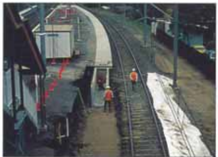
OVERALL VIEW OF APPLICATION – UNITS LAID ON SAND BED, THEN PARTIALLY BACKFILLED. NOTE CURVED PLATFORM.
