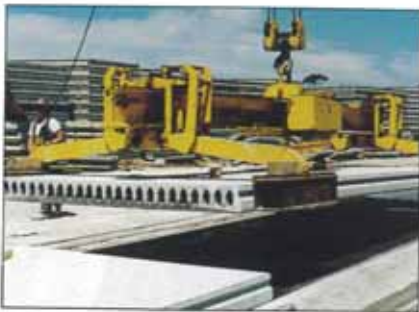
YESTERDAY'S HOLLOW CORE PANEL CASTING BEING LIFTED FROM THE BED AFTER SAWING INTO THE REQUIRED PANEL LENGTHS
