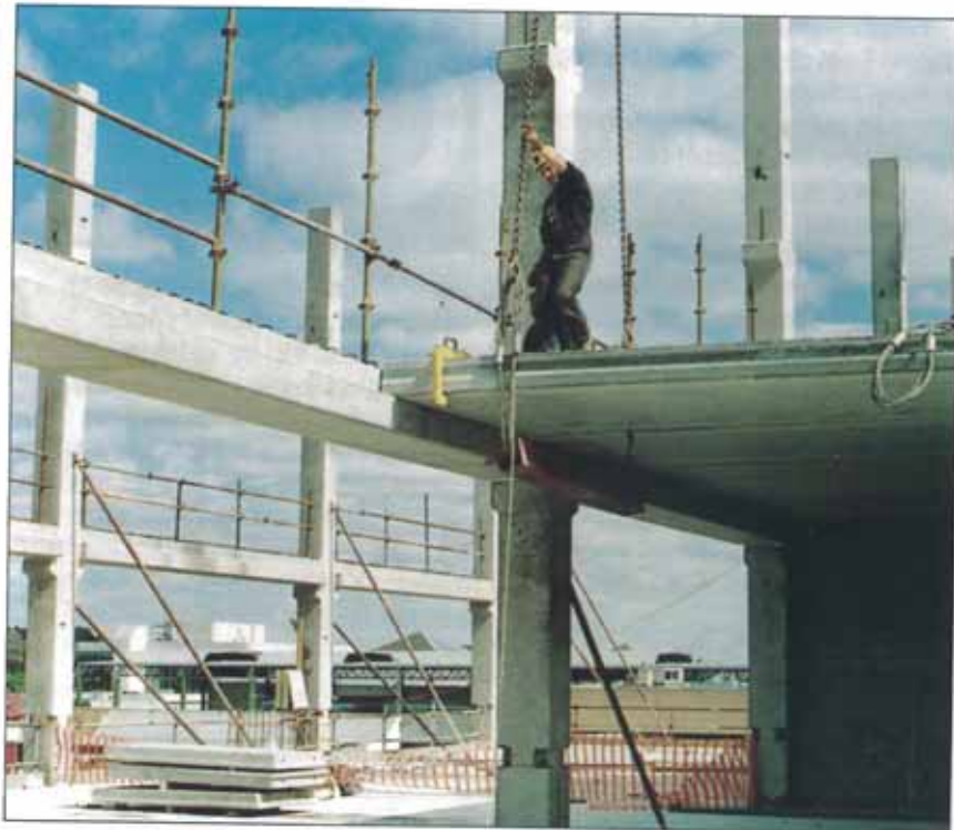
NINE-STOREY STRUCTURAL PRECAST FRAMED BUILDING WITH 33 000 m 2 OF HOLLOW CORE FLOORING – BY AUSCORE
