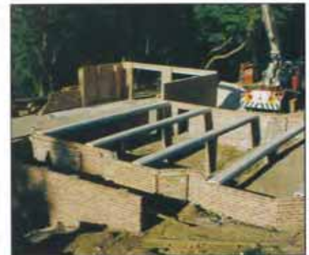
RESDEK BEAMS ON ENGAGED PIERS WITH INTERMEDIATE PIERS AS REQUIRED BY SPAN AND SPACING.
