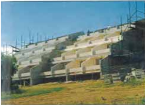
7.5-m HC PLANKS SPANNING TWO OCCUPANCIES, UTILISING PLANK PROPERTIES. NOTE USE OF HC PLANK AS BALCONY PARAPET WALL.
