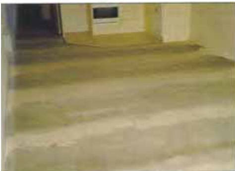
THIN COATING OF A PROPRIETARY SELF-LEVELLING COMPOUND AT PANEL JOINTS WHERE THIN, FLEXIBLE FLOOR COVERINGS ARE USED.
