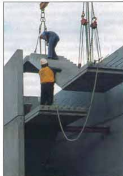
LOCATING PRECAST STAIR FLIGHT AND LANDING; USE ALSO OF PRECAST CORE WALLS.
