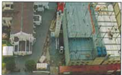
VIEW OF CONSTRUCTION IN PROGRESS. PANEL PLACEMENT RATES WERE IN THE ORDER OF 1000 m 2 /DAY.
