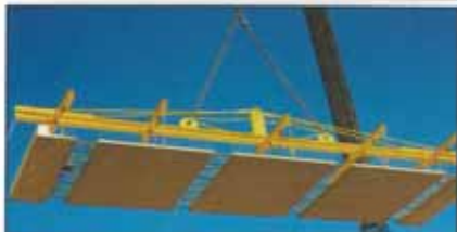
TRANSFLOOR PANELS AWAITING DELIVERY TO SITE (top) AND BEING LIFTED INTO PLACE.
