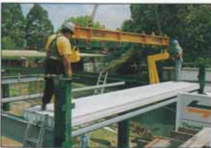
PLACING 1.2-m-WIDE HOLLOWCORE PANELS. NOTE USE OF PURPOSE-MADE LIFTING FORKS AND PERSONNEL SAFETY ARRANGEMENTS.
