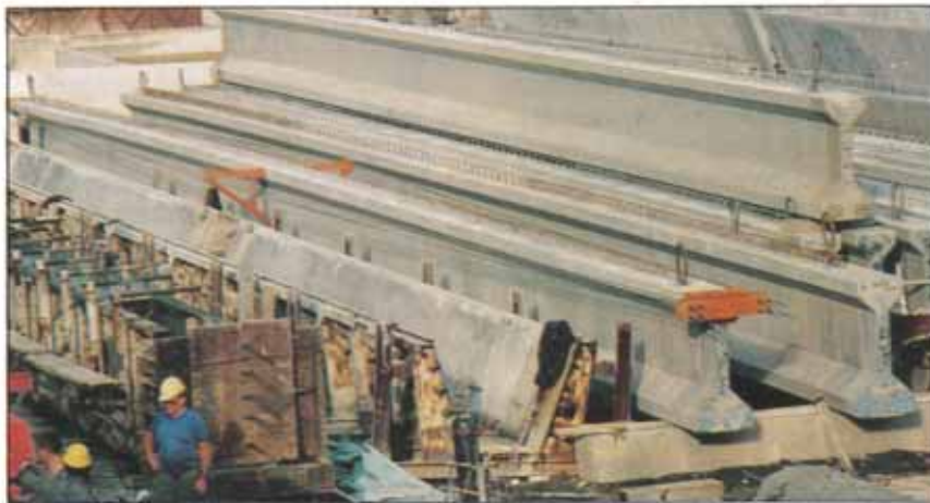
35-m-SPAN, TYPE 4 GIRDETS EXHIBITING THE BEST COLOUR CONTROL LIKELY TO BE OBTAINED ON SUCH LARGE MEMBERS.
