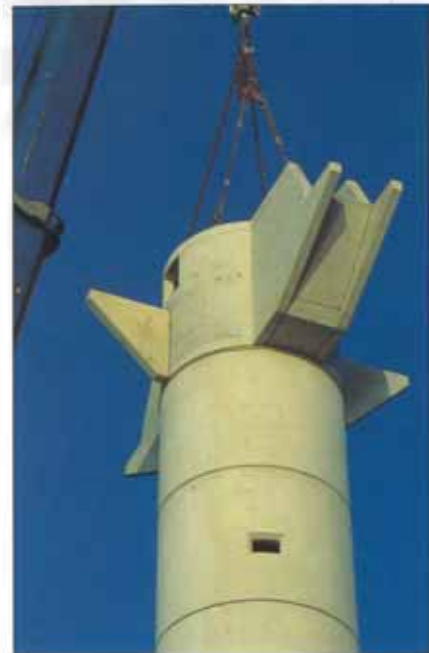
SYDNEY AIRPORT RADAR TOWER: PLACING THE FINAL SEGMENT, PRECAST DECK STILL TO BE LIFTED.
