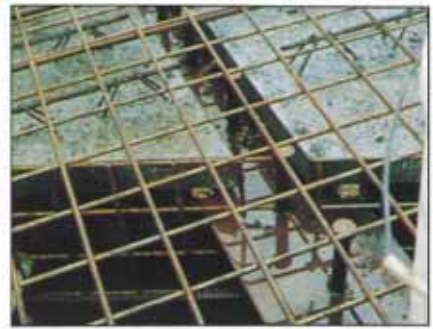
CLOSE-UP SHOWING 55-mm-THICK PRECAST SOFFIT PANELS SUPPORTED ON STEEL (OR PRECAST) BEAM.
