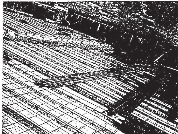
▲ Immediate and safe working platform provided. Note top reinforcement prestressed by welding to cast-in trusses.
